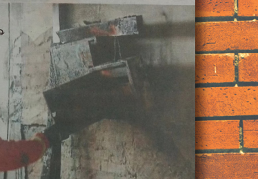
Totally destroyed: A fireman looking at the charred fuse box in the main switch room of SMK Tongod. - Photo courtesy of fire department
